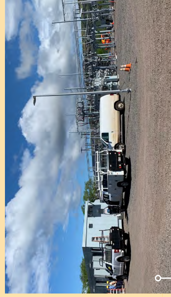
Construction on a new substation at the Pacific Missile Range Facility is completed, allowing for full output from the AES PMRF solar+storage facility
