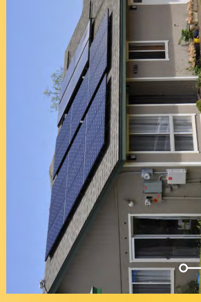
358 new photovoltaic installations are completed so far in 2020
