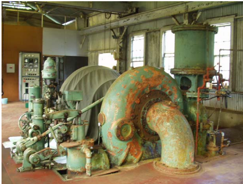
Figure 8-6. Lower Lihue Plant 800 kW Turbine.
